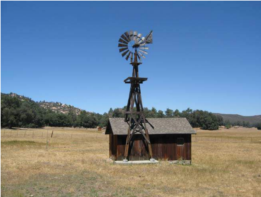
This windmill and pumphouse are used to supply water to *****
