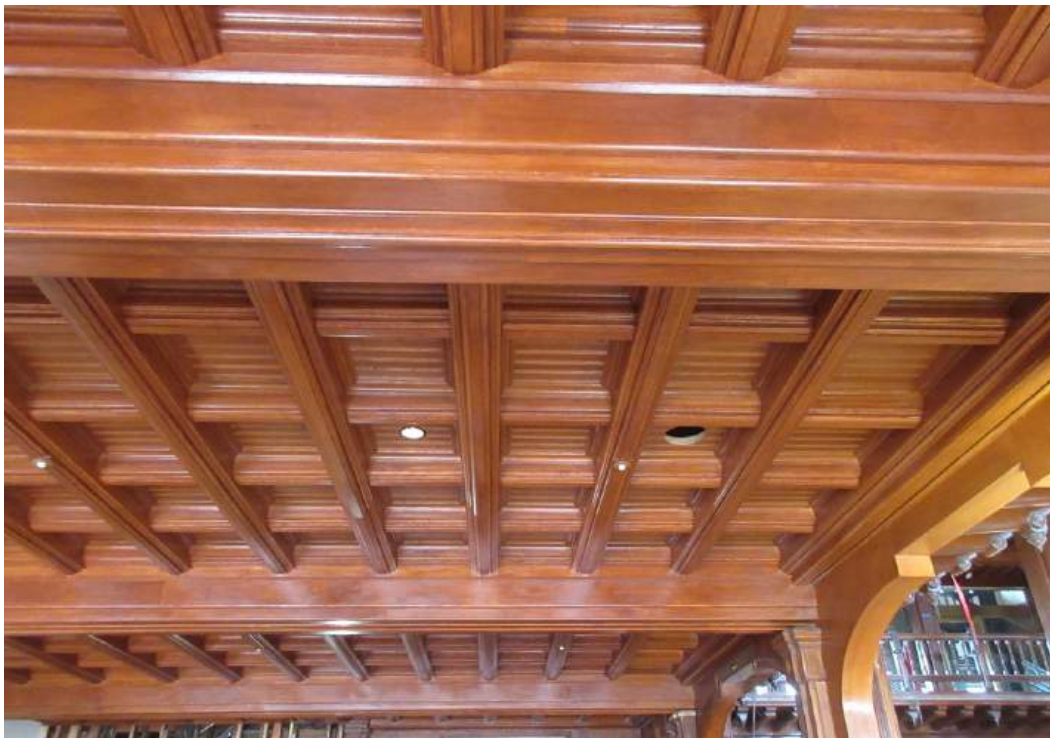
Figure 35: The original reassembled coffered ceilings are the two furthest bays. The two nearest bays are new coffered ceilings where the Front Desk area was expanded. The white dots under the beams are recessed sprinkler heads.
