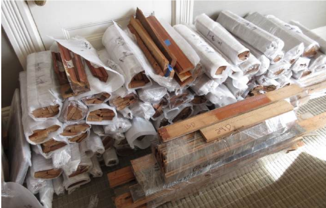
Figure 34: The Front Desk coffered ceilings needed to be dismantled and salvaged to install new structure, electrical and fire sprinklers. Here the labeled coffers are being stored in a guest room.
