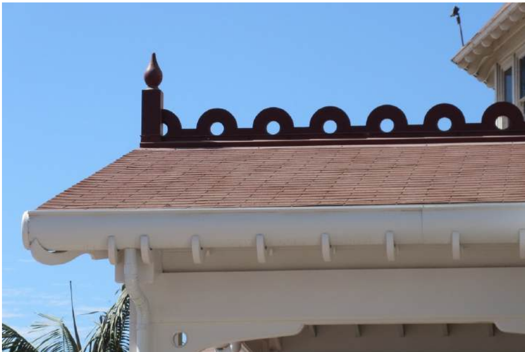
Figure 51: The missing ridge cresting at the gable roofs was recreated from historic photos using durable PVC with mahogany finials.
