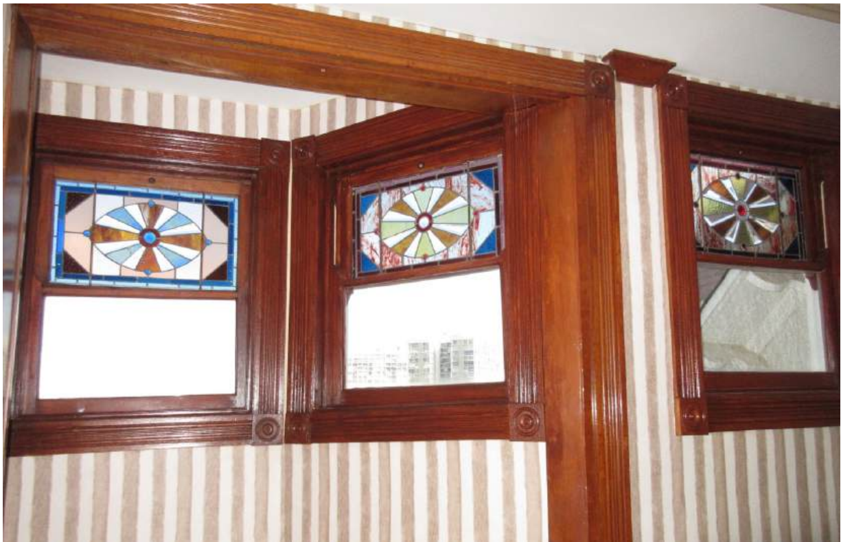
Figure 64: Three historic stained-glass windows at the third floor west stairwell were restored and reinstalled. Two missing adjacent windows with the same design are being fabricated.
