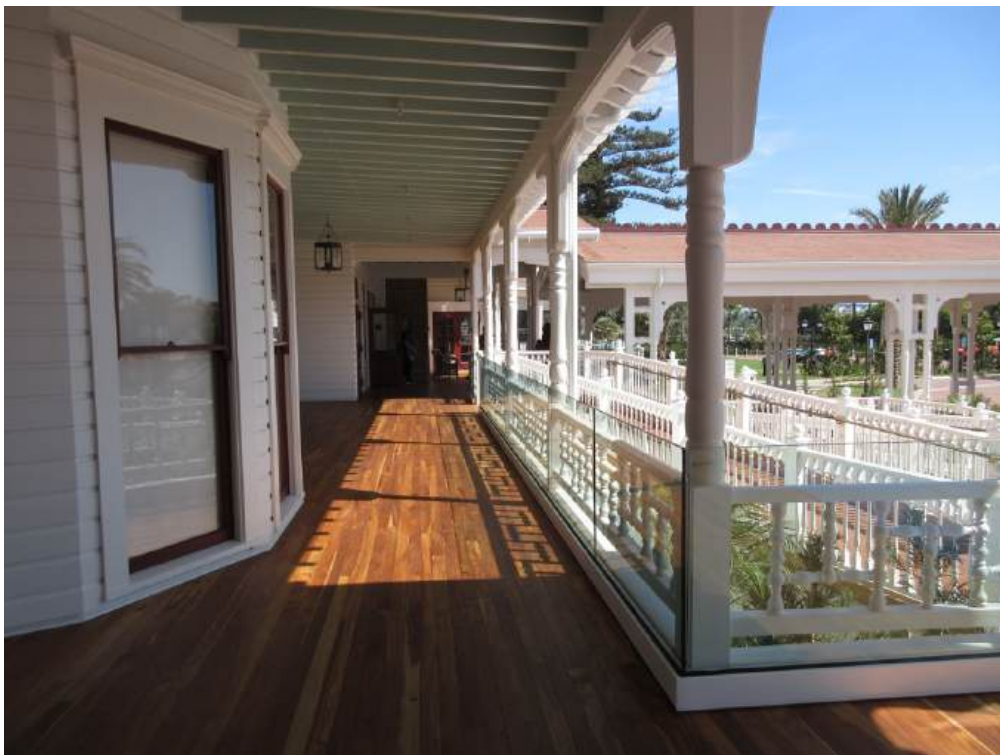
Figure 92: After - Same view (believe it or not) after restoration, 9-23-21. The location of the railing is where the south wall had been located.
