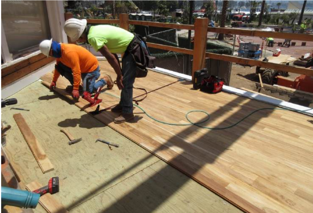
Figure 44: T&G teak flooring being installed over plywood at the east end of the Veranda.
