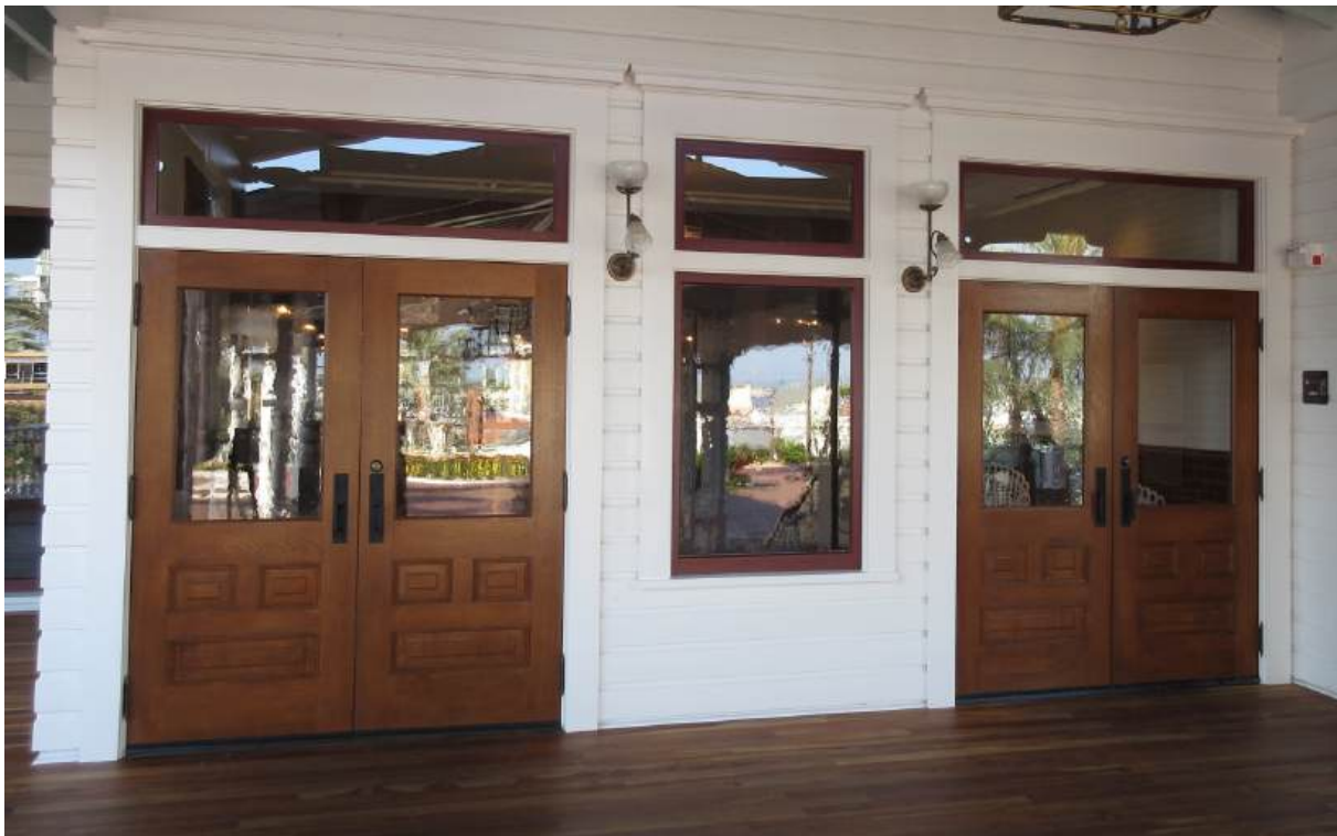
Figure 59: Replica white oak panel doors at the main entrance with a stain and shellacked finish and Victorian reproduction bronze hardware. The doors were widened to 36-inches to comply with the ADA. The stained-glass transoms are not yet installed.
