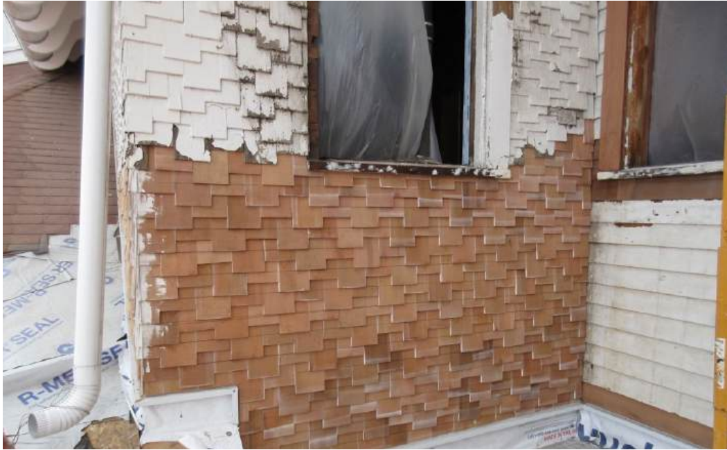
Figure 54: A dormer on the west side of the second floor shows a mix of original wall shingles (upper) alongside replicated cedar wall shingles (lower). Also note the shiplap siding on the right.
