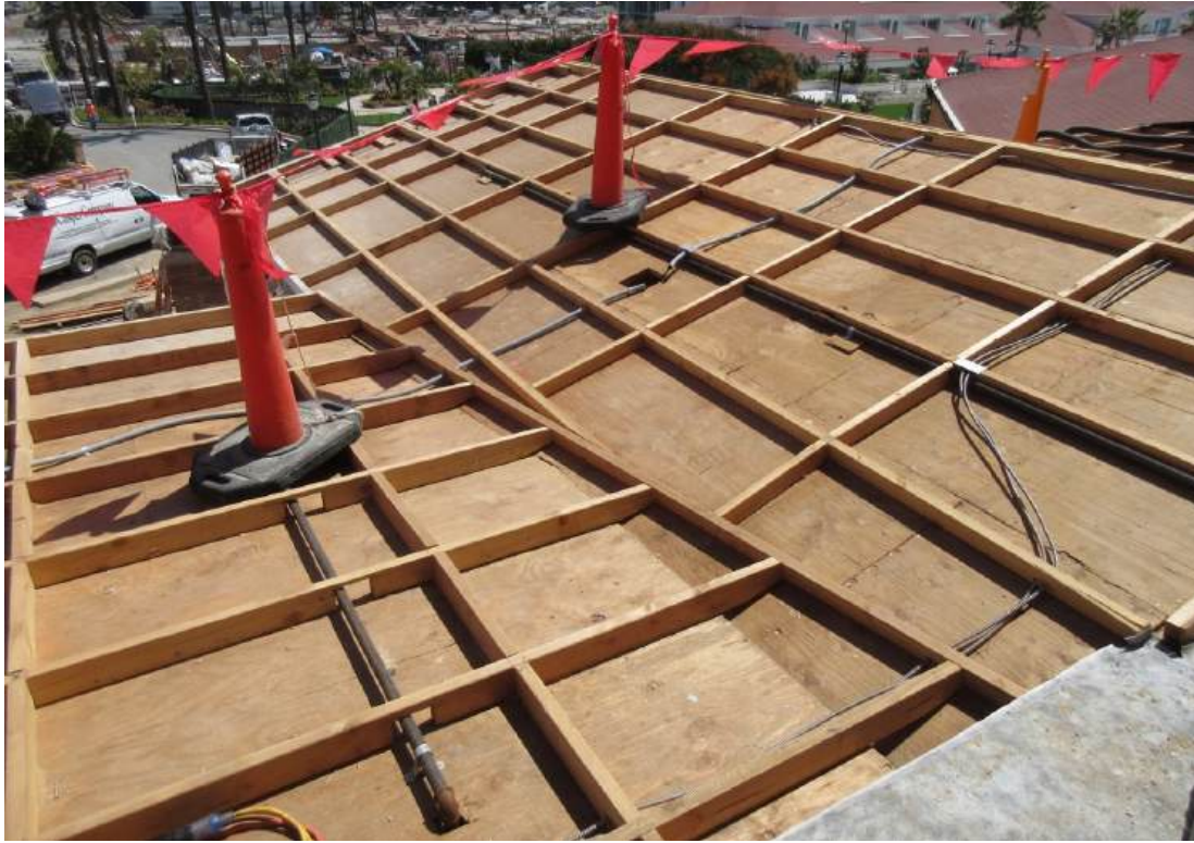
Figure 42: This “sleeper space” above the Veranda ceilings provides room to conceal fire sprinkler pipes, electrical conduit and speaker wires that would otherwise be exposed.
