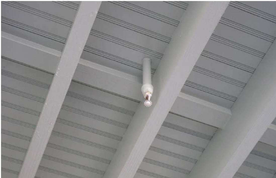
Figure 43: View of the Veranda ceiling showing that only the sprinkler heads are visible. Fire codes require that the heads extend past the bottom of the roof joists.
