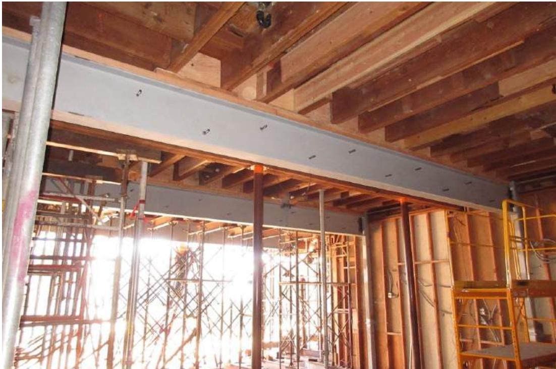
Figure 33: New steel beams were added above the Front Desk area to allow two non-historic pipe columns to be removed.
