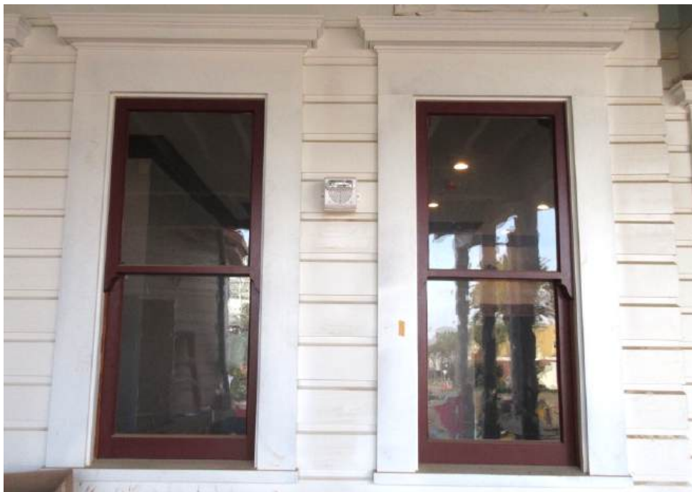
Figure 57: Replica double-hung windows and trim at the Veranda. The “ogee lugs” are the curving extensions of the sash frame that are on all of The Del’s original window sashes, upper and lower.
