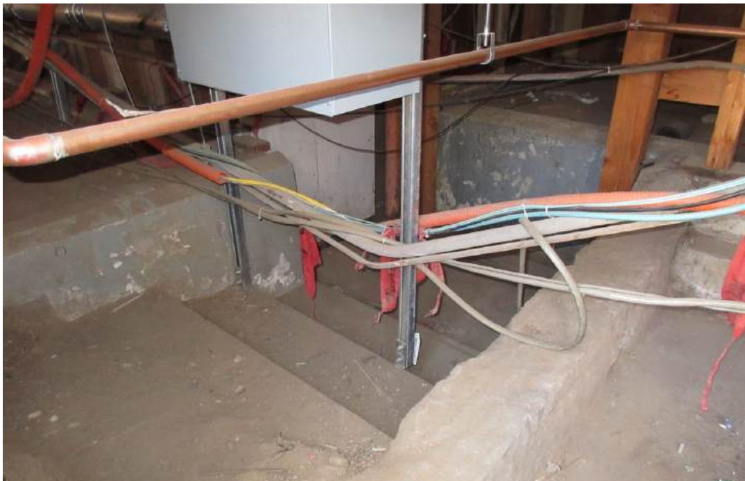
Figure 23: The original concrete Barber Shop stairs are extant in the crawl space below the previously extended Veranda. These will be left in-place.
