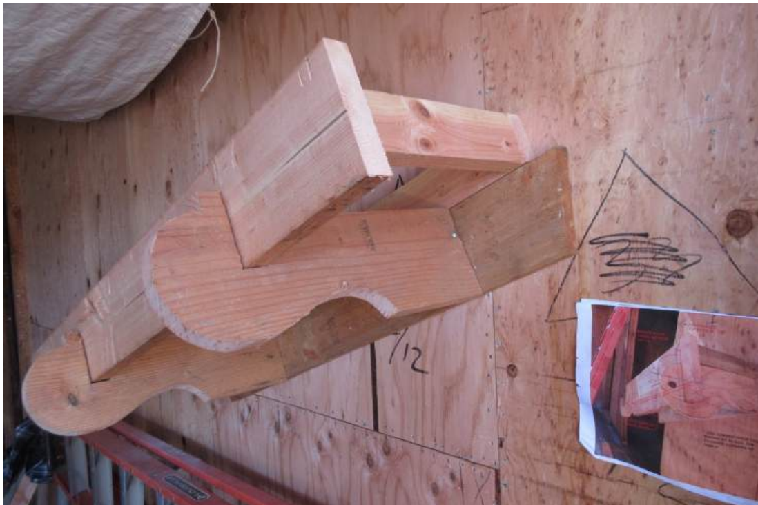
Figure 25: This mockup was created to review the shape of the rounded rafter tails to show how they met the fascia board at the main entry roof gables. Note the marked-up photo on the right.
