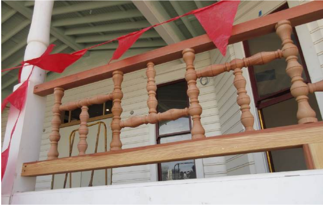
Figure 52: Newly fabricated mahogany guardrails at the Veranda that exactly match the historic detailing, prior to being painted.
