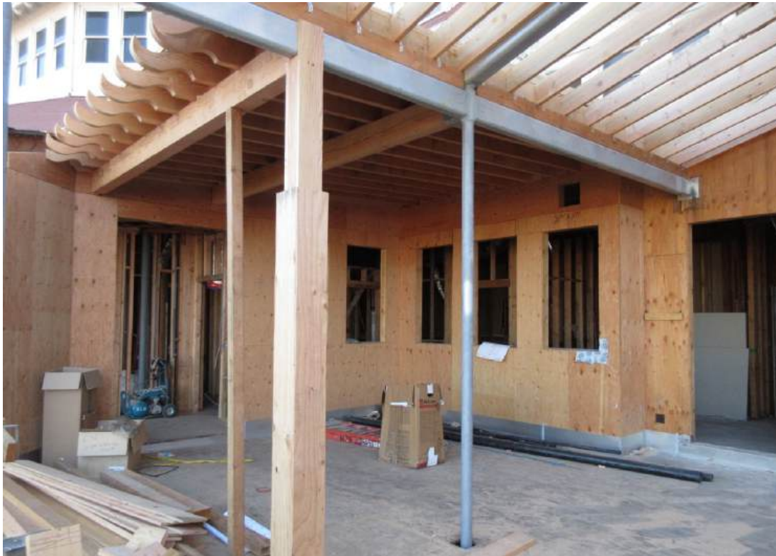
Figure 46: The original Veranda was all wood construction, but the restoration required the incorporation of steel framing and fasteners to meet structural requirements.
