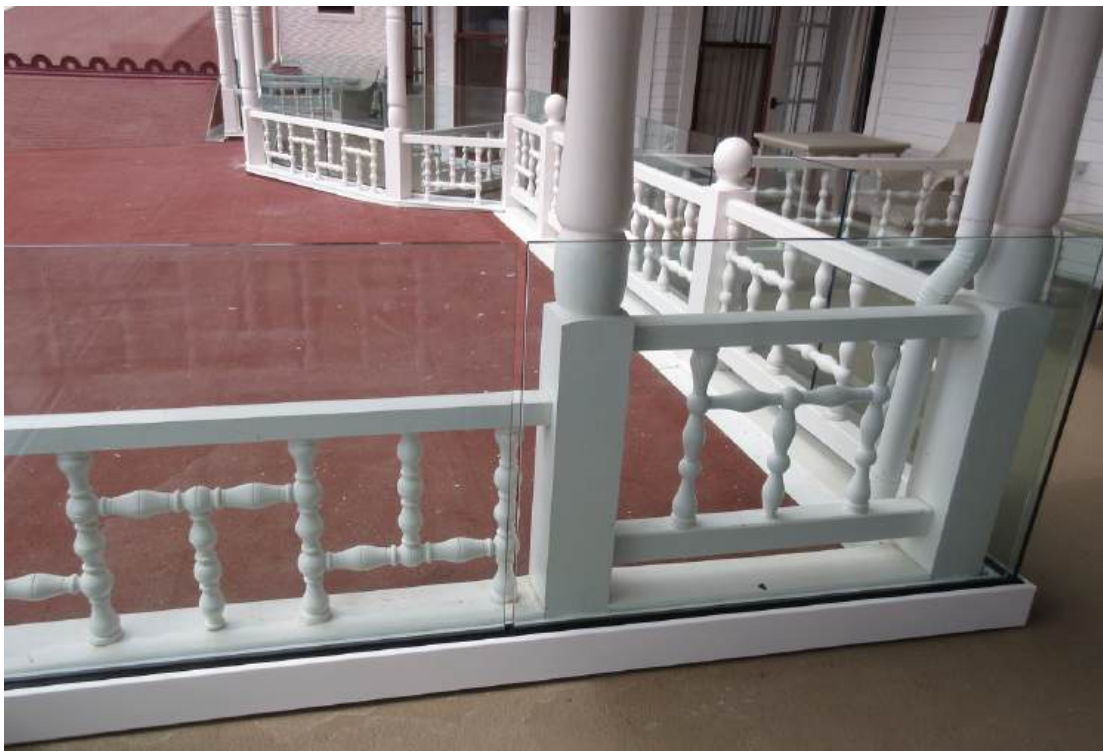
Figure 53: Simplified guardrails without the groove details (on the right) were installed in areas where railings did not historically occur in order to be differentiated per The Standards . Frameless glass guardrails were added on the back side to comply with code requirements.
