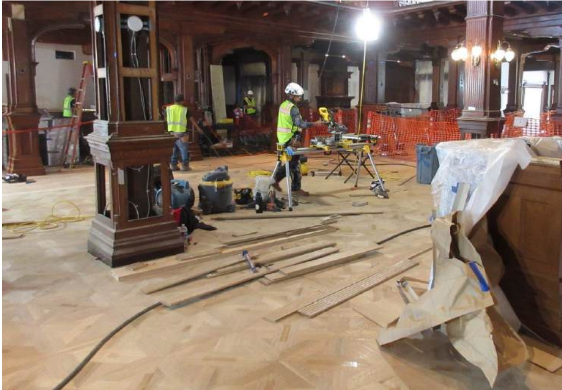
Figure 32: New oak flooring being laid. The center of the Lobby has a diagonal pattern and two-tone border. Refer to Figures 38 and 39.
