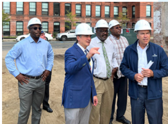
Knox Building, Springfield, Massachusetts. Mayor Domenic J. Sarno, Chief Development Officer Tim Sheehan, State Representative Bud Williams, and Ward 5 City Councilor Lavar Click-Bruce joined Gordon Pulsifer, President of First Resource Development Company, for a tour of the redevelopment of the historic Knox Building. The redevelopment and construction project will yield over 100 new affordable apartments. According to Mayor Sarno, “My administration is proud of the continued investment and development in our neighborhoods utilizing vital state and federal historic tax credits.” COURTESY CITY OF SPRINGFIELD, MASSACHUSETTS
