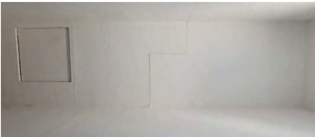
Figure 15 - Cracking of stair ceiling between main level and upper level. Cracking is indicative of building movement/settlement.
