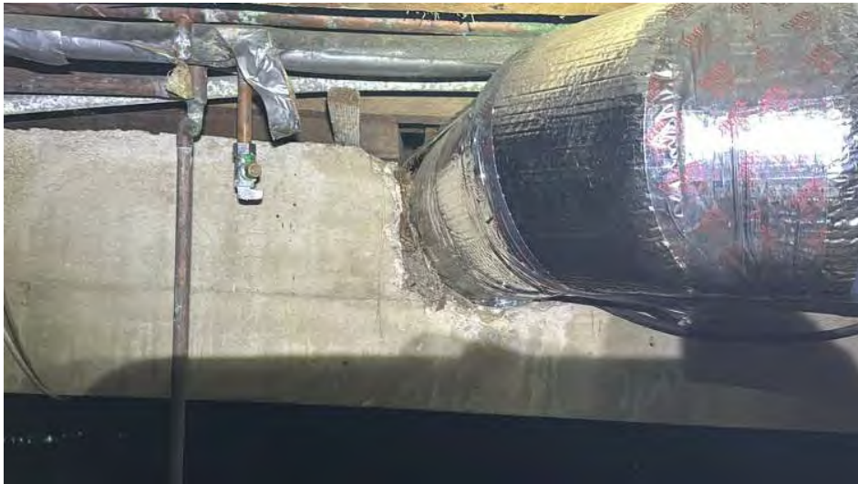
Figure C - Notch in foundation beam to accommodate ductwork.
