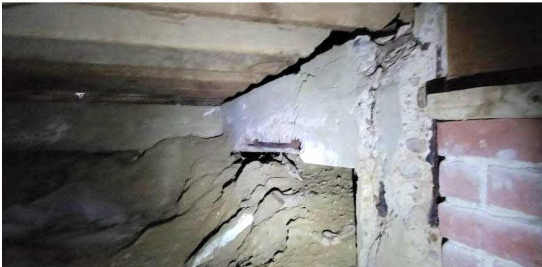
Figure 11 – Opposite Side of Column shown in Figure 10 showing substantial deterioration.
