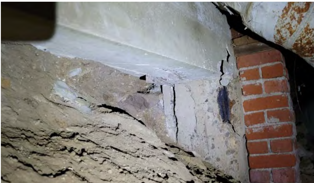
Figure 9 – Rebar Corrosion, Cracking and Spalling in Concrete Column and grade beam at North Wing. Note that both corners are spalling substantially as is blind side of beam.
