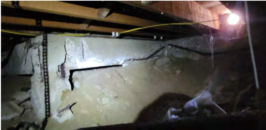
Figure 13 – Grade Beam and column showing significant deterioration. Reinforcement in corner has corroded and is completely broken.
