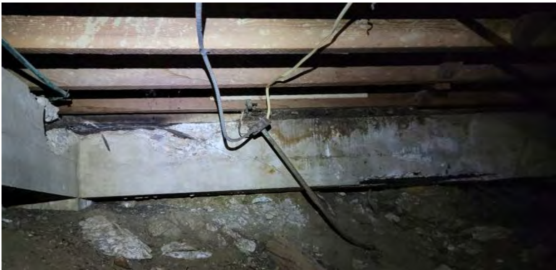
Figure 1 – Rebar Corrosion, Cracking and Spalling in Concrete Grade Beams at South Wing
