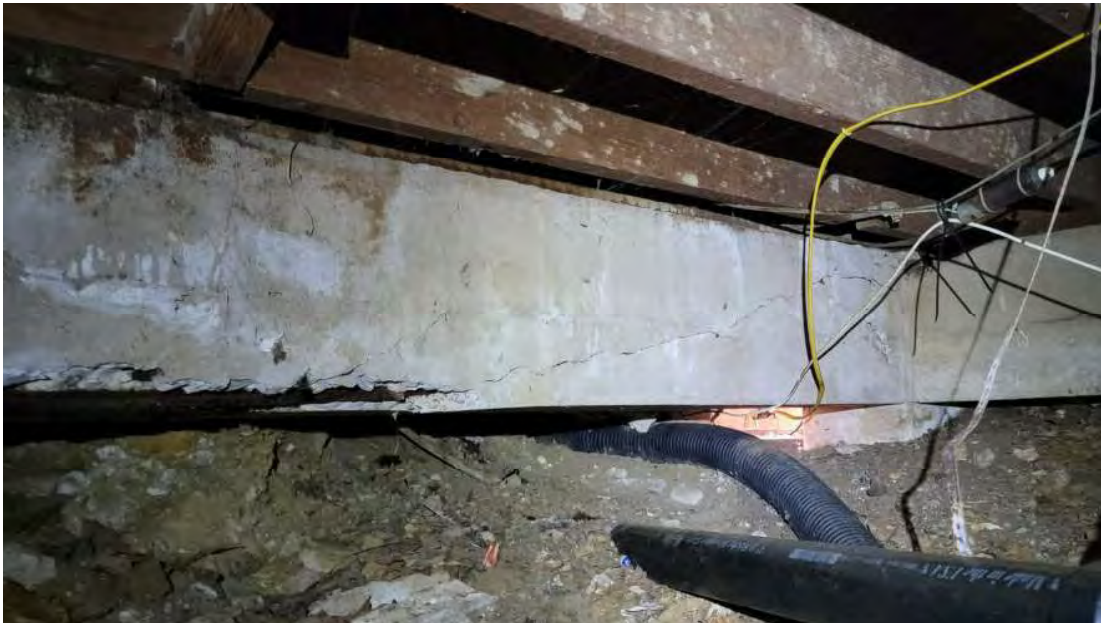
Figure 3 – Substantial Diagonal Crack (Shear), Spalling of Concrete, Corrosion of Rebar in South Wing Grade Beams.
