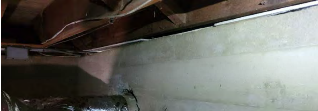
Figure 6 - West wall of South Wing, Wall on right slopes down towards the west with gap size increasing to the west. West portion of building appears to have settled and been shimmed to re-level structure above.
