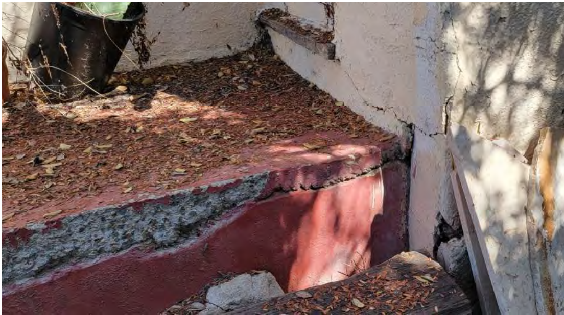
Figure 8 – Exterior Patio Area and Surrounding Walls Cracking and showing signs of settlement/distress.
