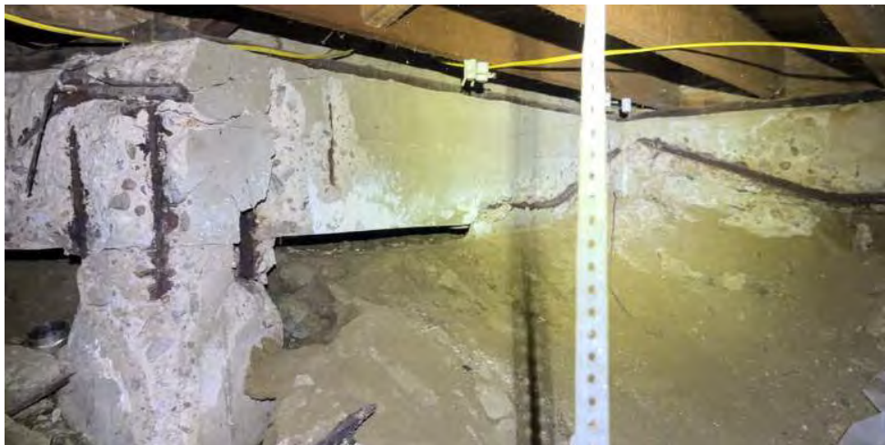
Figure A - Rebar Corrosion, Cracking and Spalling in Concrete Grade Beams at Western Portion of Building
