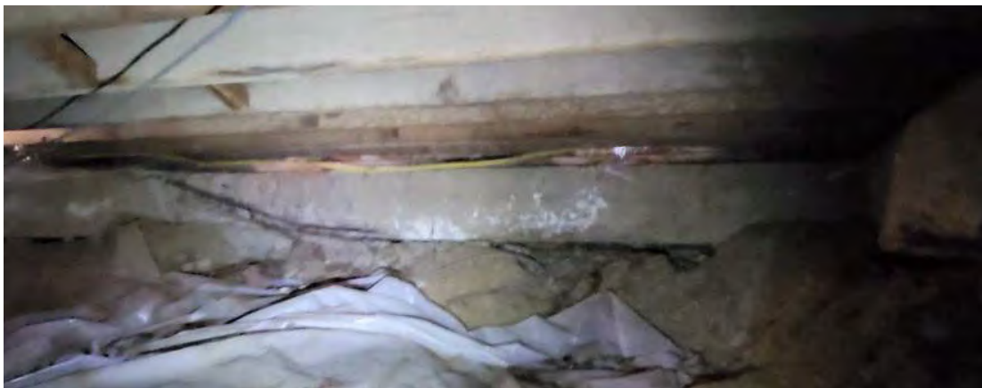
Figure 12 – Grade Beam showing deterioration and flexural failure and deflection.
