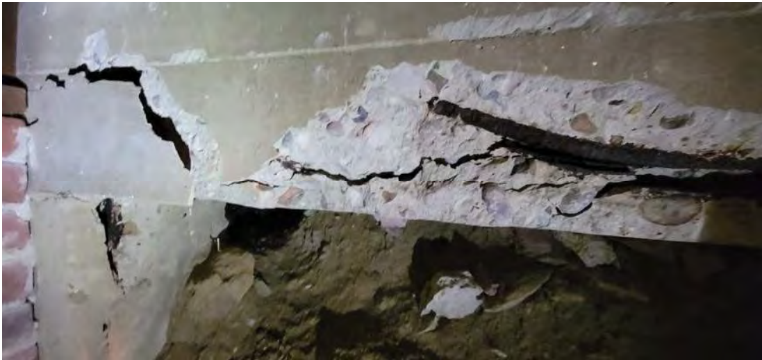
Figure 10 – Opposite End of Grade Beam shown in Figure 9 showing substantial spalling and corrosion
